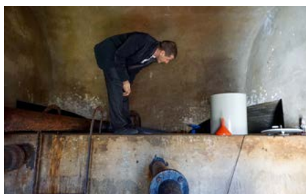
A Swiss expert inspecting the drinking water reservoir built in 1960 in the Croatian municipality of Fužine. © SECO
