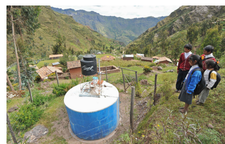
Drinking water chlorination system approved by SABA. San Salvador district, Cusco region. Photo: SDC
