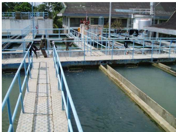
The restored water purification plant in Lambaro (Banda Aceh) supplies the inhabitants with drinking water. © SDC
