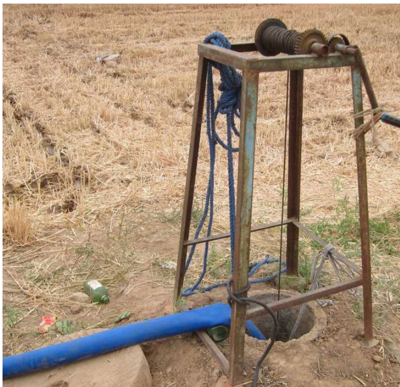
Submersible groundwater pump tapping aquifers for irrigation in Guantao County © Pedrazzini 2015
